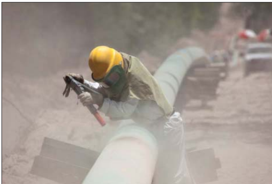
A worker helps construct the Arbuckle Pipeline, a 440-mile natural gas liquids pipeline extending from southern Oklahoma through the Barnett shale of North Texas and on to Mont Belvieu, Tex., on the Gulf Coast. Construction was completed on the line in late July. Photo from Oneok Partners.
