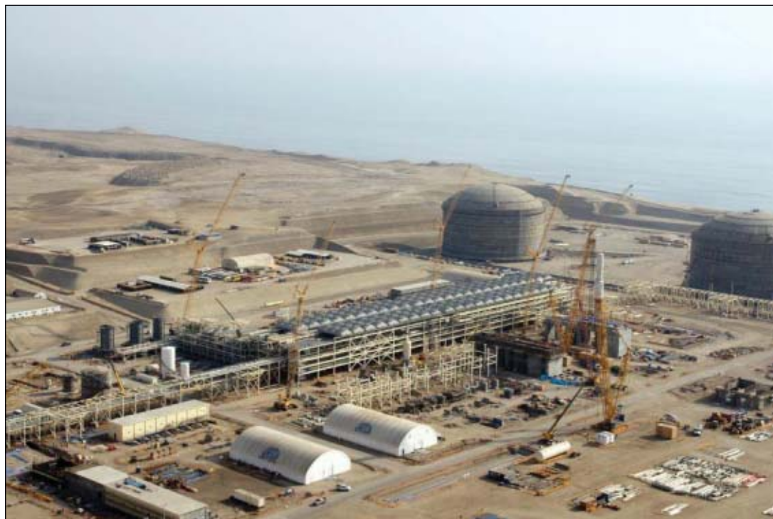
The Peru LNG liquefaction plant is not only the largest industrial project ever to be undertaken in Peru, but is also South America's first baseload LNG export facility. CB&I was awarded a contract for the engineering, procurement, fabrication, construction, and commissioning of the plant in January 2007. Completion is slated for 2010. Photo from CB&I.
